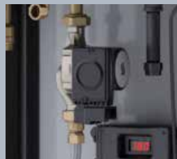
High Flow Recovery Pump
